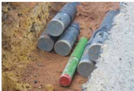
150km cabling in ducts, and a control building is built to connect the wind farm to the existing power grid.
