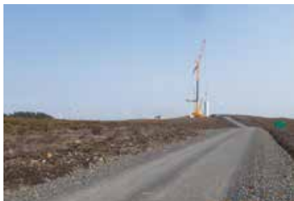
Each turbine component lifted into place using two cranes – three tower sections, the hub, nacelle and blades.
